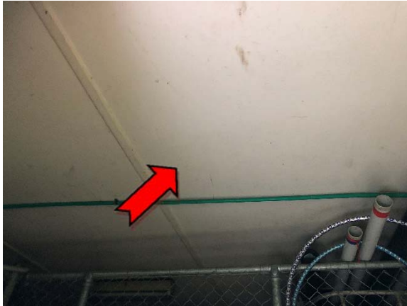
Photo 1. Interior, store room, ceiling – asbestos-containing fibre cement sheeting.
