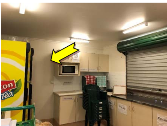
Photo 5. Interior, kitchen, walls, throughout – suspected lead-containing cream paint system.
