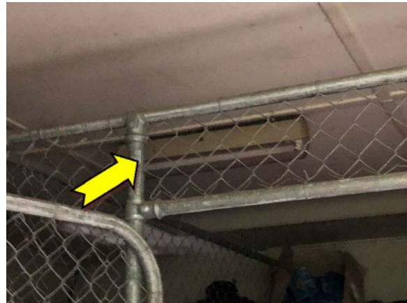
Photo 4. Interior, throughout, single tube fluorescent light fittings – suspected PCB-containing capacitors.
