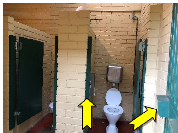
Photo 6. Interior, male and female toilets, doors and door handles, throughout – suspected lead-containing green paint system.
